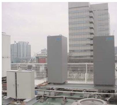
Fuel cell power systems mounted atop building in Shinagawa, Tokyo, Japan are providing combined heat and power for occupants as part of an ongoing fuel cell demonstration project.
